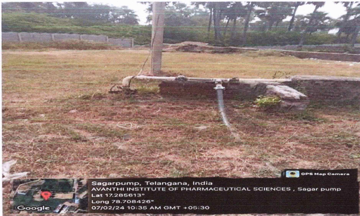
7HP Motor capacity was installed opposite to girls hostel
