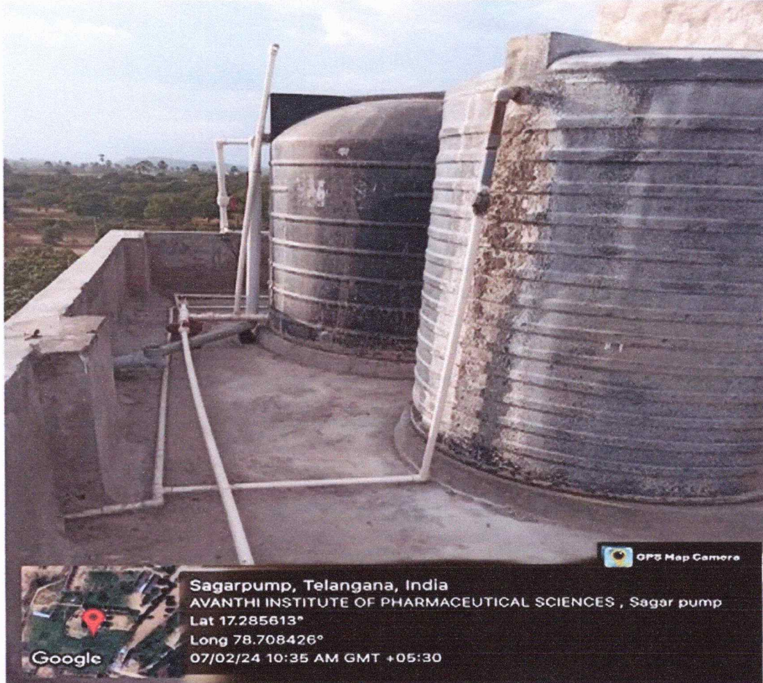
Top UP of Pharmacy Block SYNTEX Tanks of capacity 2500 liters of each
