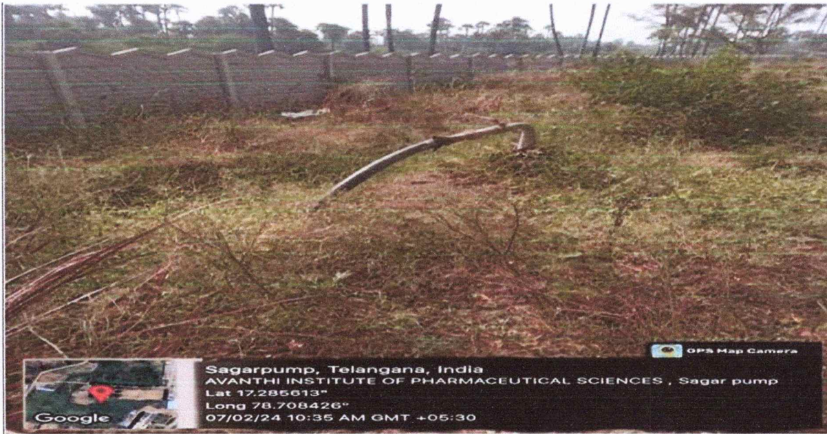
7 HP Motor capacity was installed near the Near Pharmacy Block
