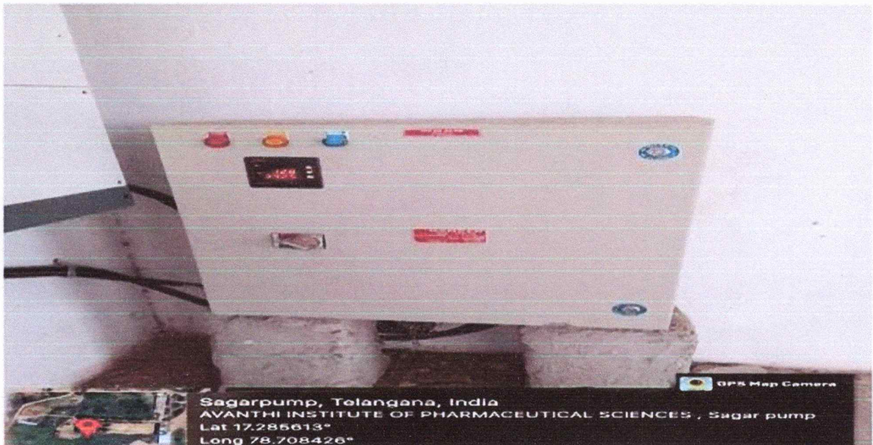
Solar plant connected to power grid
